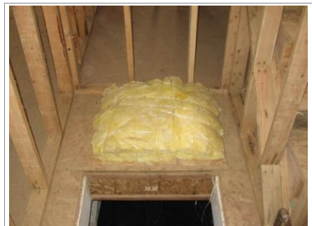
R402.2.4 Access Hatches and Doors Insulated crawl space access. The same method applies to attic access hatches
