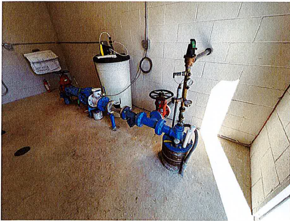
SR505 Well House Interior
