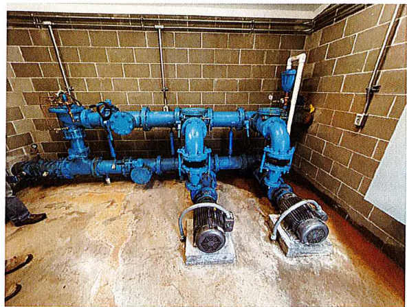
Eureka Booster Pumps
